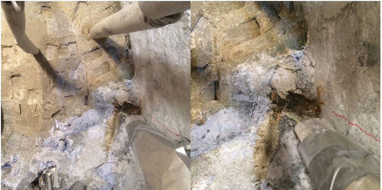
Fig. S36-6: Corrosion halos above of cable duct to the right (3 o'clock).
