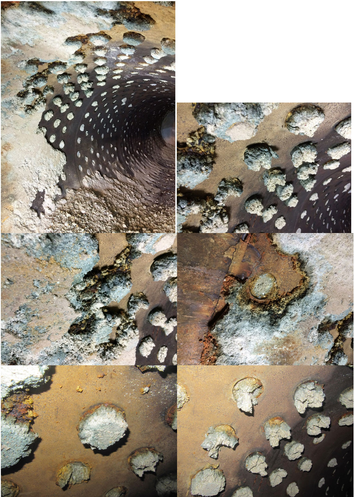
Fig. S42-5: Corrosion halos/features at bentonite protrusions inside the liner.
