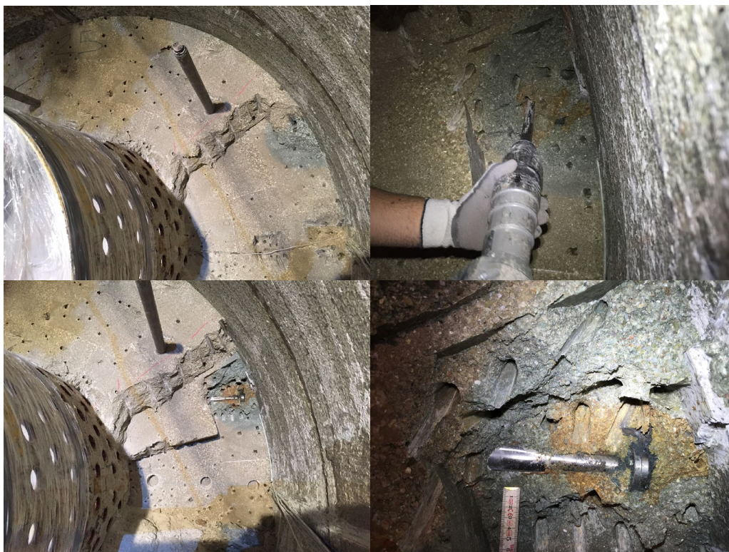
Fig. S54-2: Corrosion halos when approaching and during dismantling of displacement sensor S-S-54-15 (see for more information in NAB 16-054).
