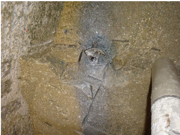
Fig. S42-8: Discolorations in front of an abandoned drill bit (see more details in Section 44).
