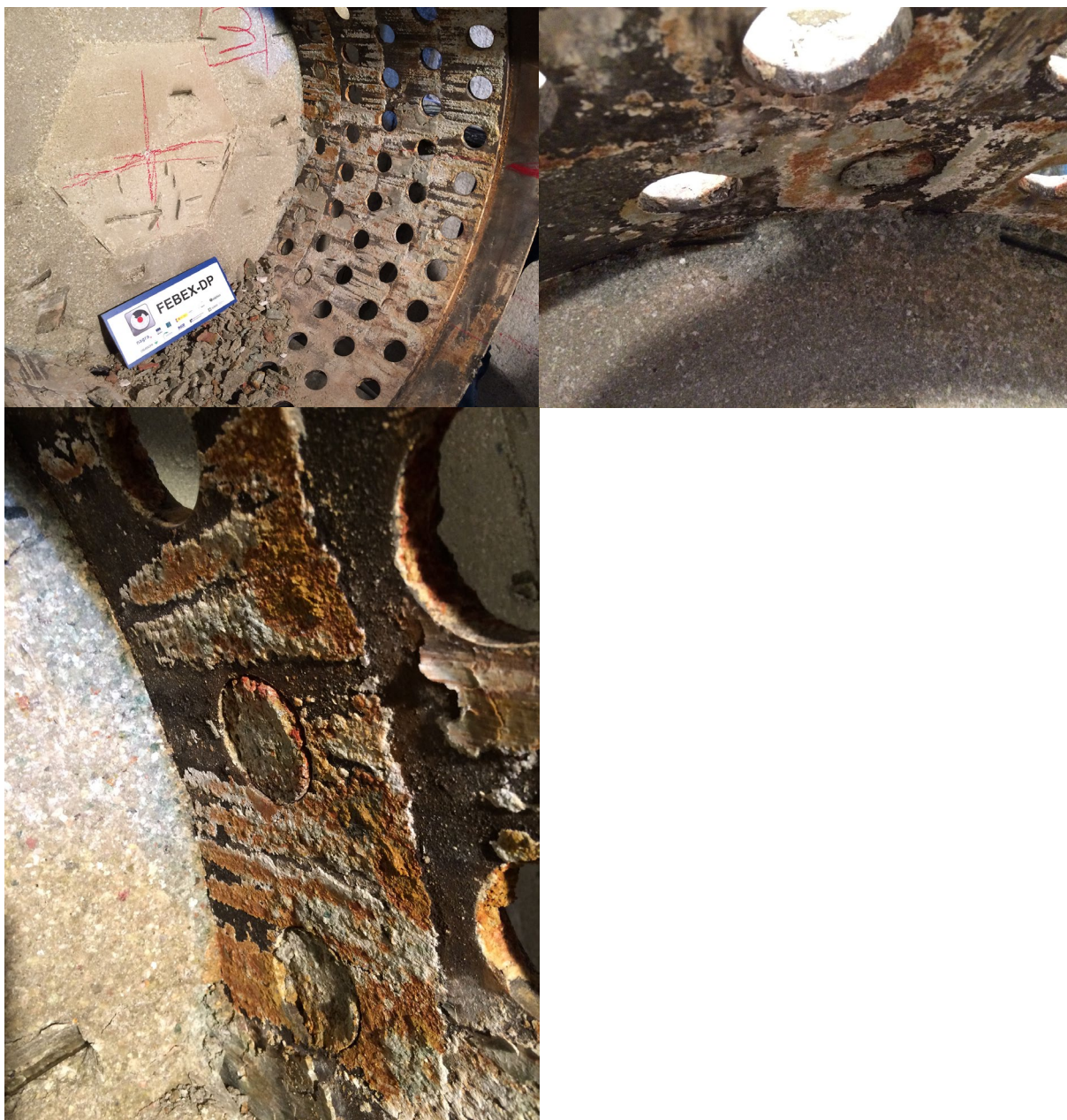
Fig. S41-6: Corrosion features inside the liner.
