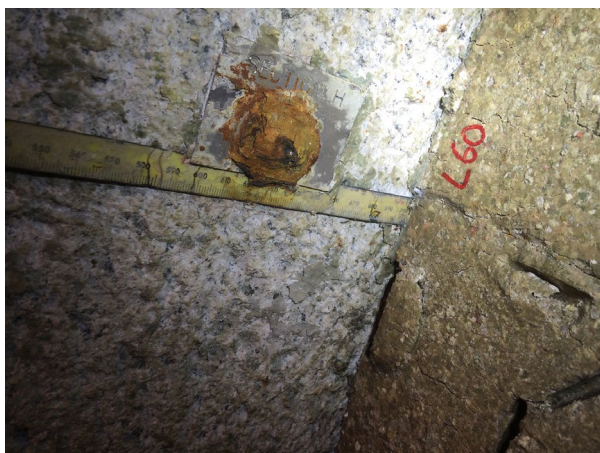
Fig. S42-2: Corrosion of a leftover metal anchor in the granite wall.
