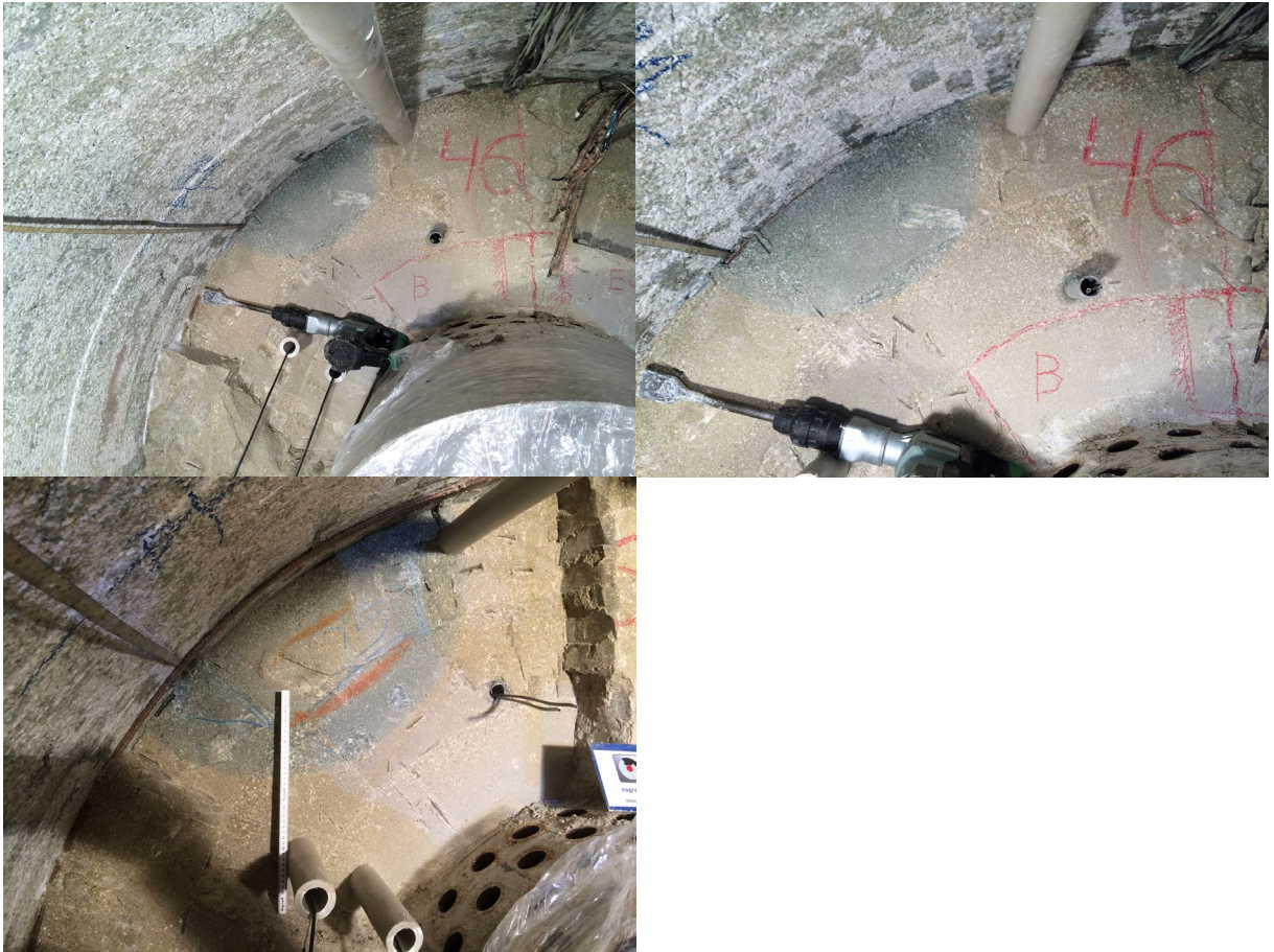
Fig. S46-3: Bentonite discoloration related to the corroding fisurometer (see further details in Section 47).
