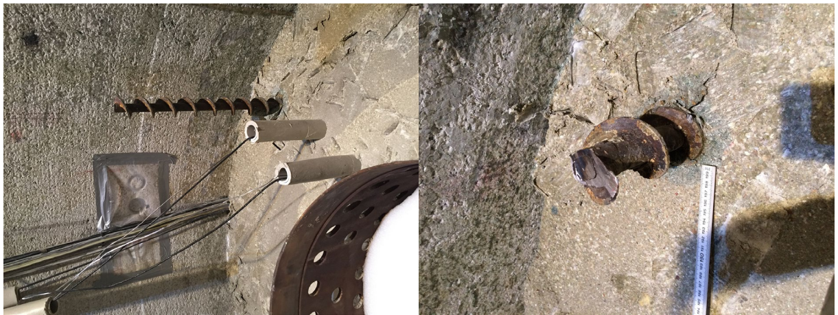
Fig. S44-2: Discolorations surrounding an abandoned drill bit. Drilling and bit were abandoned due to drilling problems during the partial dismantling in 2002 when further gas-water pipes were installed.
