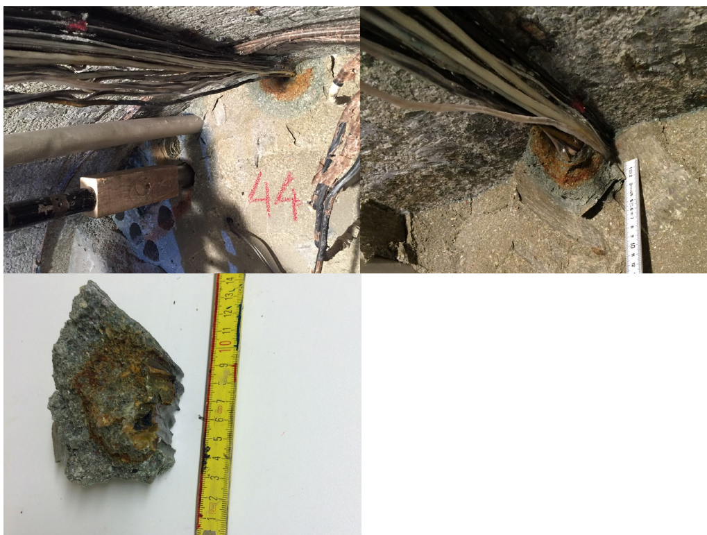
Fig. S46-2: Bentonite discoloration halos surrounding the roof cable duct and a piece thereof that was in contact with the bentonite.
