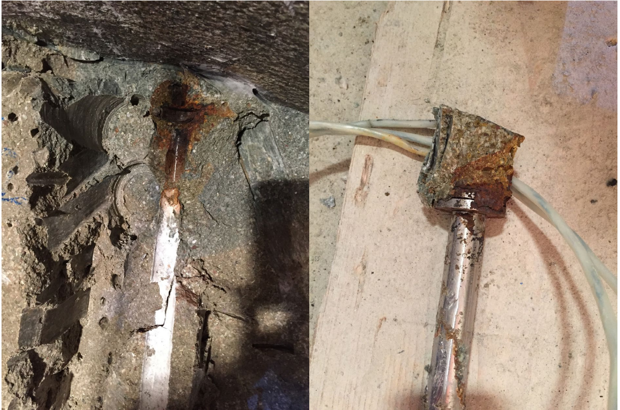
Fig. S54-3: Corrosion feature around displacement sensor S-S-54-14 (see NAB 16-054 for more information).
